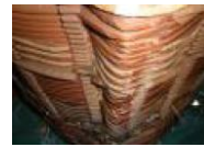
Fig. 1. Typical winding buckling failure, [2].
